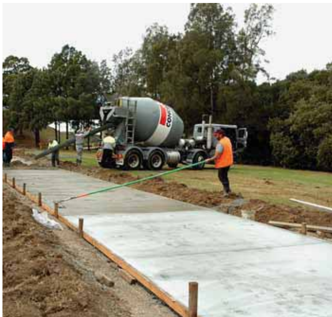
Funding capital projects including footpaths and shared cycle routes continues to be a major component of Council's annual capital expenditure (David Wallace Photography)
