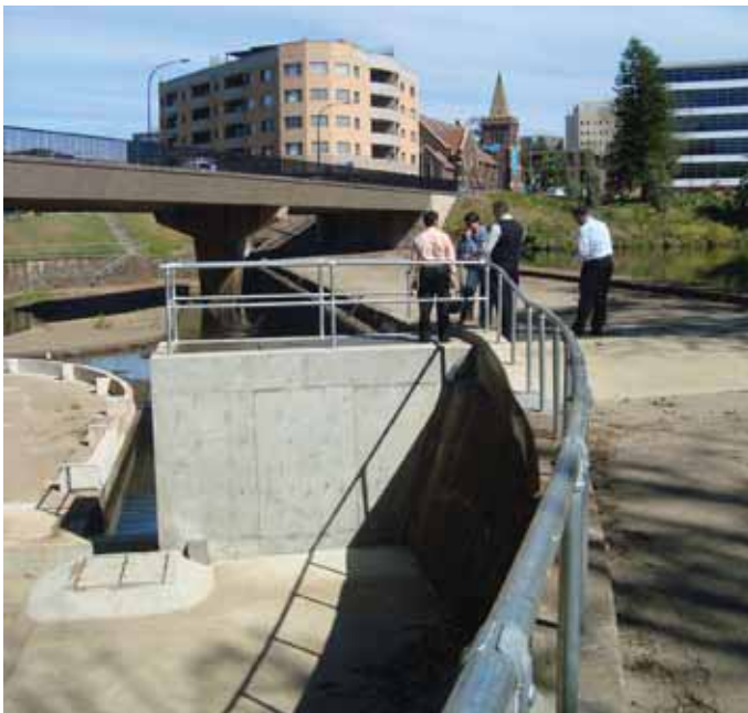
The rectangular structure is an innovative engineering solution that assists native fish to circumvent the Marsden Street weir and travel upstream to feed and spawn
